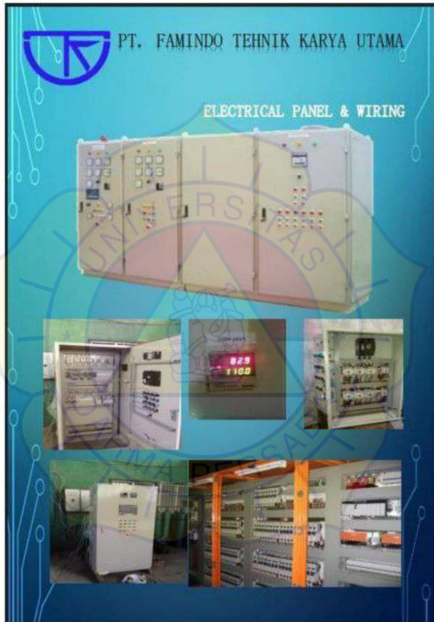
Lampiran A. 1 ELECTRICAL PANEL & WIRING
