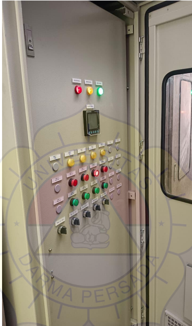
Tampilan Luar panel PLC Control Cooling tower
