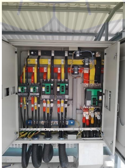
Gambar 2.22 Panel AC Combiner (Cikarang Listrindo, 2024)
