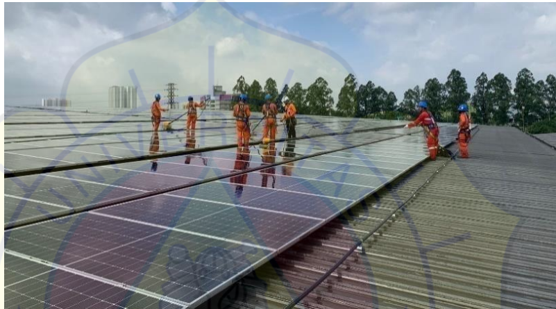
Gambar 2.14 Perawatan Panel Surya
